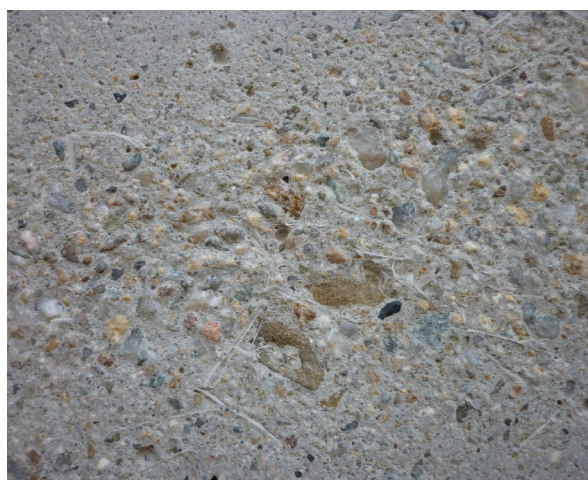
Figure 7 – The surface of the concrete sample micro-reinforced with steel fibers ZS/N – 0,50x30mm: 1 – fiber indentation, 2 – fiber cutting
