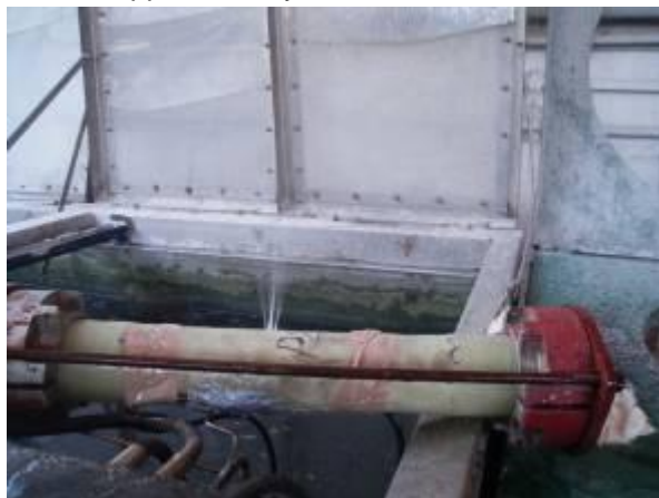
Figure 4 - Start of the pipe leakage
