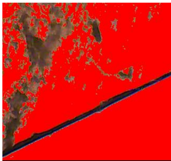
Figure 9. Modified image of Fig. 5. for easier detection of damaged structure in the quantification process.
