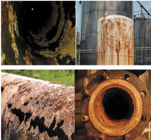
Fig.2. Different forms of Corrosion [45]
